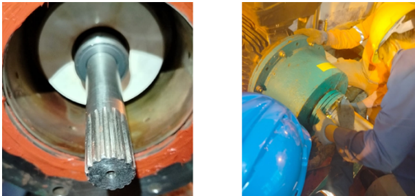
Figure 1. HP Pump SWRO UBP Labuhan Angin (Source: Private archive, 2025)
